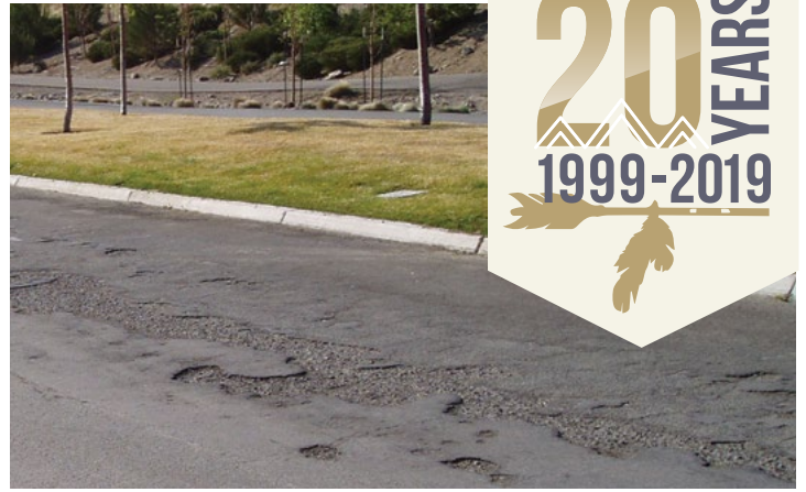
Pothole arising from prolonged moisture exposure
