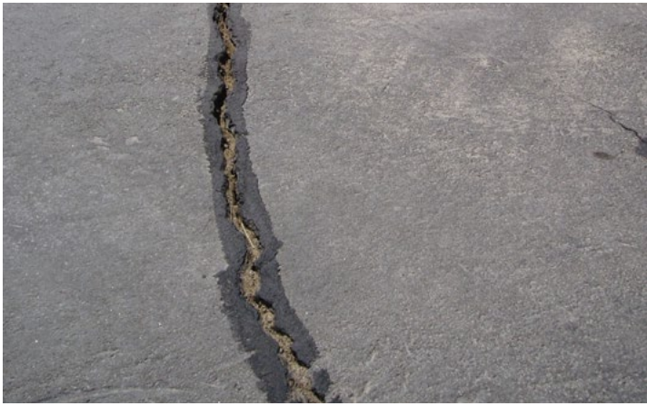
Premature transverse crack
