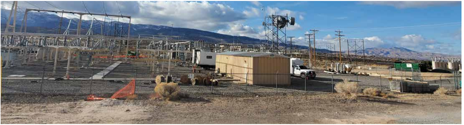
This is the substation that services ArrowCreek. ArrowCreek is straight back in the photo.
