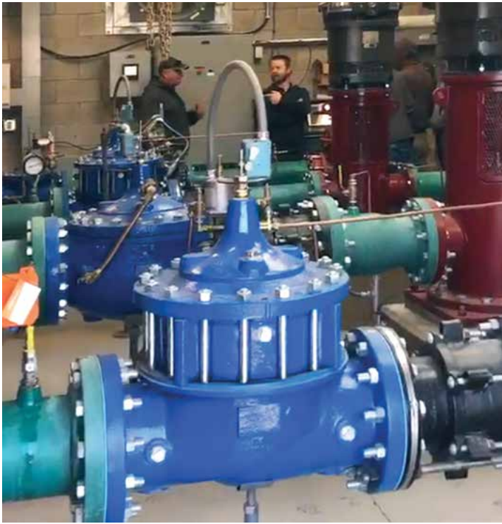
Truckee Meadows Water Authority technicians during a recent test of the Hunter Creek Pump Regional Station.
