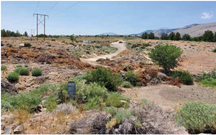
The retention basin/pond at The Pit. (Private Property of The Club at ArrowCreek)
